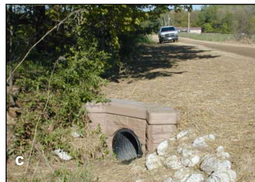
Walls can be made with a variety of materials including native stone (a), boulders (b), or molded plastic (c).
